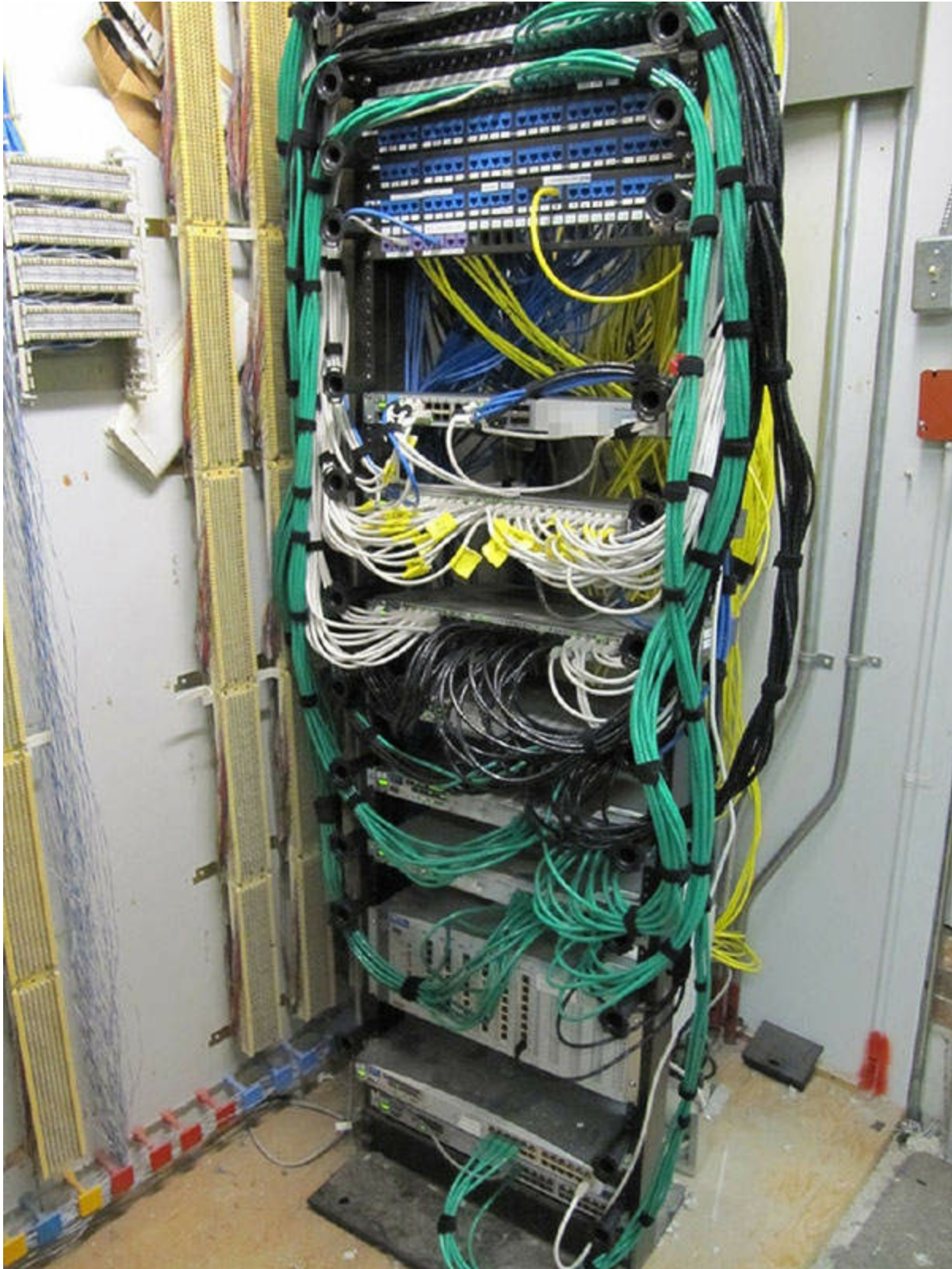
FIGURE 10.1 A typical wiring closet
