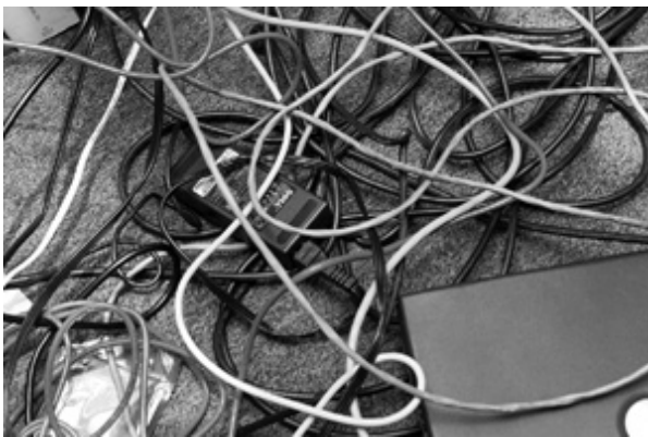
Figure 2-9 Mike's cable kludge
