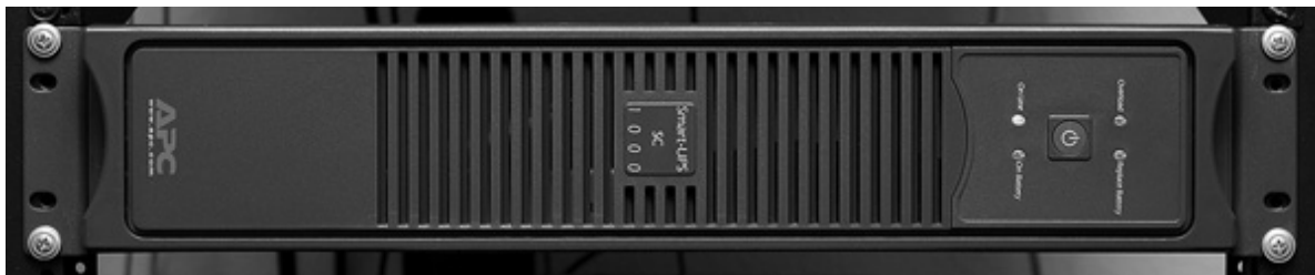
Figure 29-1 UPS on rack
