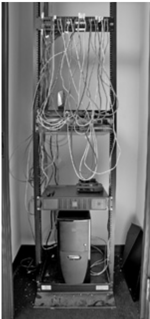
Figure 24-22 A wiring closet
