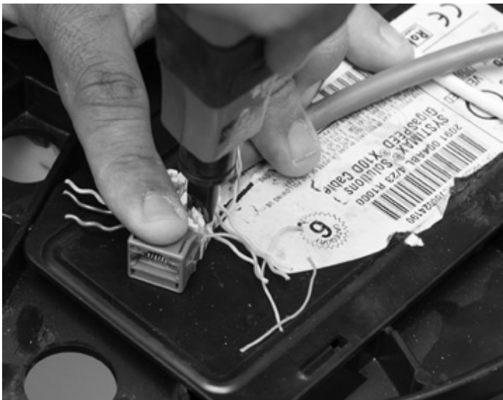
Figure 22-31 Punching down a modular jack
