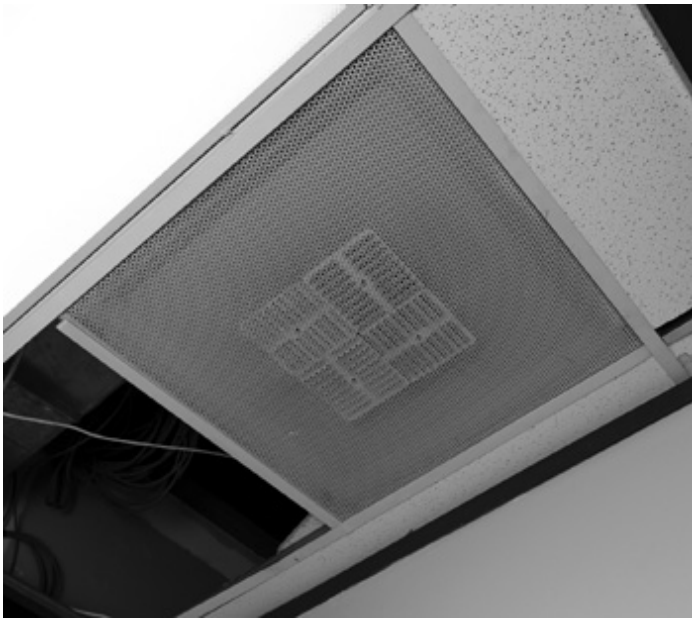
Figure 29-3 Air-conditioning vent in a small server closet
