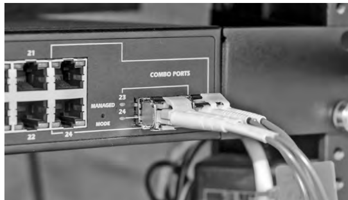
Figure 5-12 Switches with dedicated, high- speed ports
