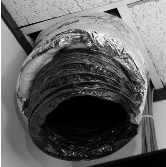
Figure 6-28 An A/C duct cooling a telecommunications room
