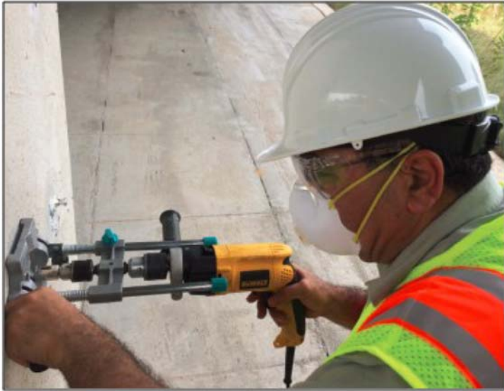
Figure 7.2 Coring FRP material around test dollies with portable drill press.
