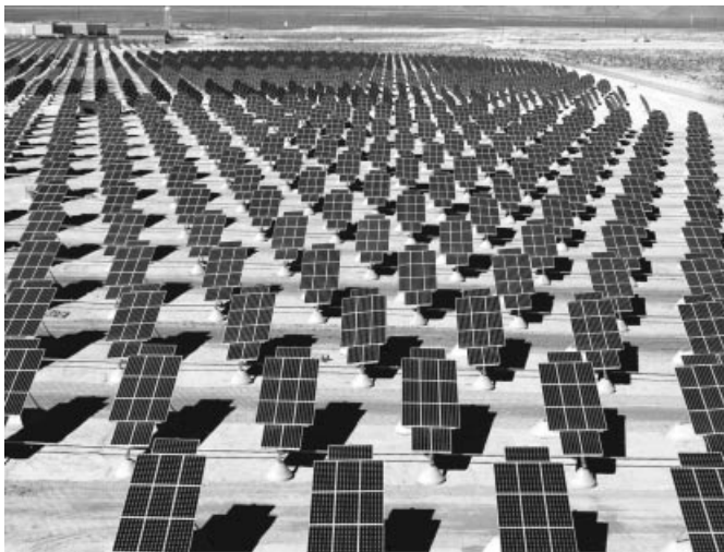
Figure 13.1 A 14 MW power plant installed in 2007 in Nevada, USA (Source: U.S. Air Force, http://en.wikipedia.org/wiki/Renewable_energy )
