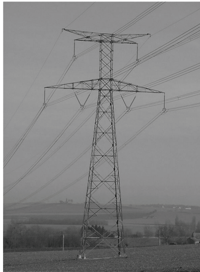
Figure 5.16. Overhead Power Lines Subject to Gallop
