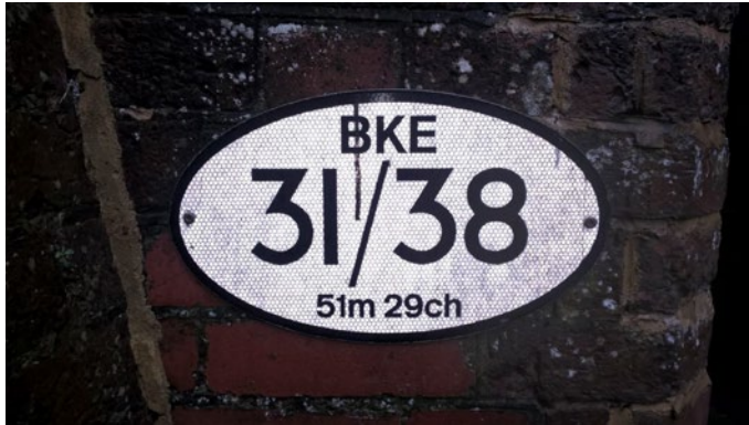
Figure 2-1. A sign identifying a British railway bridge. The figures at the very bottom represent a distance from some datum, in miles and chains
