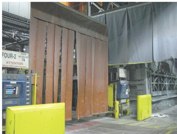
Figure 9. Protective curtains lowered at cast start-up to avoid metal projections in pedestrian zones.
