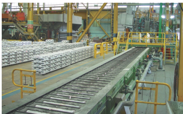
Figure 1 Typical ingot conveyor line [4].
